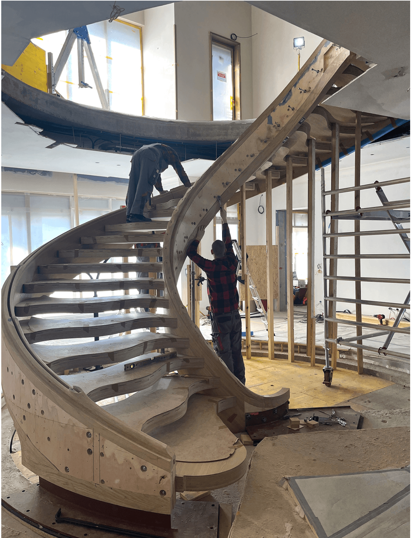
On-site installation of the primary structure, showing the integration of prefabricated elements.
